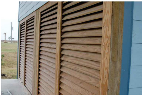
Wood louvers installed beneath an elevated house in a V zone are a good alternative to solid breakaway walls
