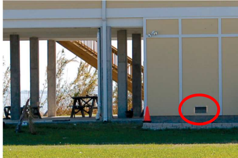
Flood opening in a below-BFE enclosure wall (A-Zone)
